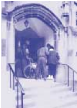
Figure 18: After nearly five years of planning and fundraising, construction has begun for a new accessible ramp and entrance. (See project drawings in Figure 17) Neal A. Vogel for Restoric, LLC
