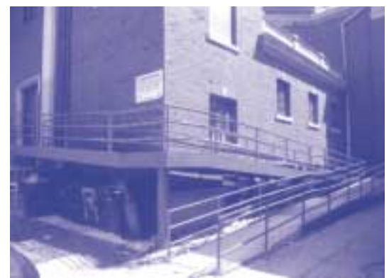
Figure 6: This ramp is too long is too steep, requires frequent maintenance (painted steel) and has an industrial appearance. Neal Vogel for Restoric, LLC
